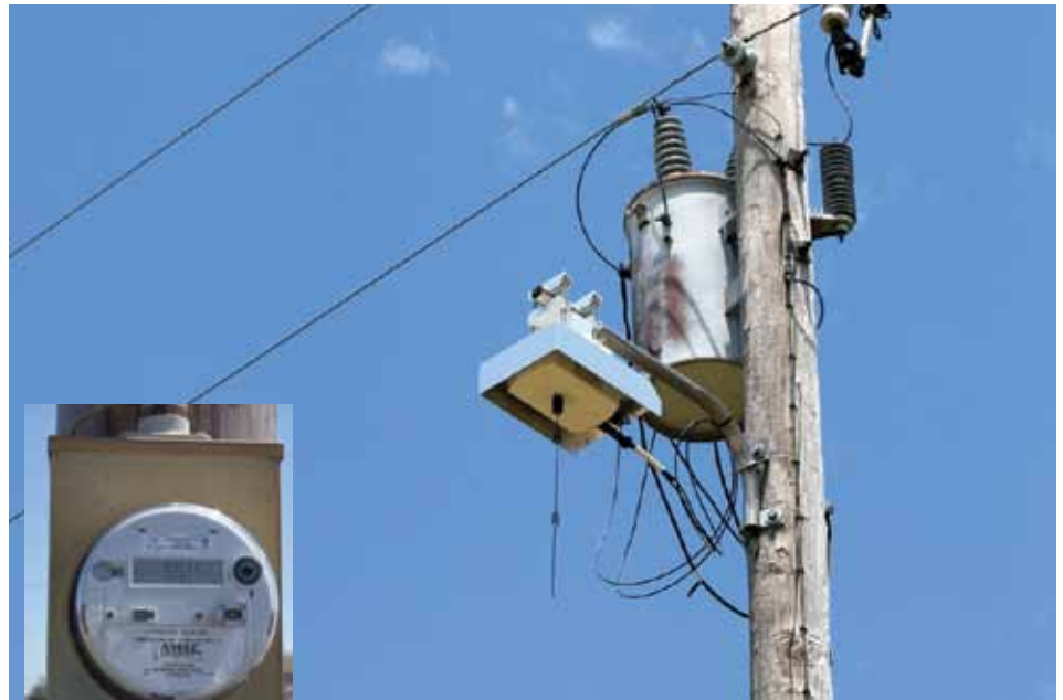
The new smart meters transmit data wirelessly in near real time via the 450 routers NWECC has strategically placed across its system.
